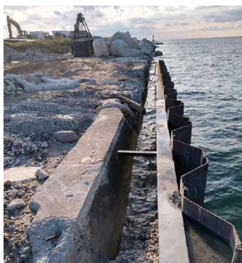
Top. New walkway caps Portage Lake’s rebuilt channel wall. Above. Old Portage Lake channel wall (at left) and the new steel wall, under construction.
