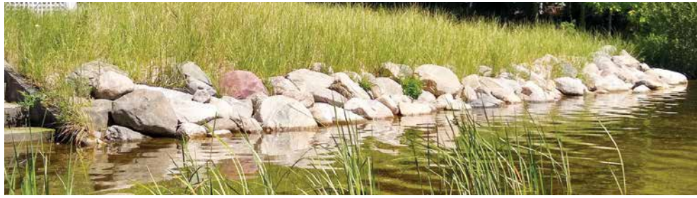
Riprap (in this case, rocks), with spaces for vegetation, and beach grass are considered good ways of preventing erosion, while still allowing habitat at the shoreline. Photo by S.A. McFerran.
