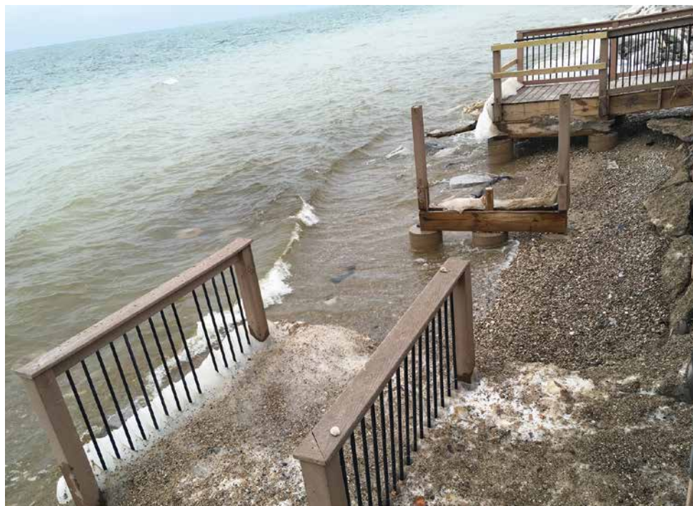
Bar Lake Outlet’s viewing platform was recently shored-up by steel, but the wheelchair ramp and stairs to the beach were destroyed by waves. Photo by Pat Stinson.
