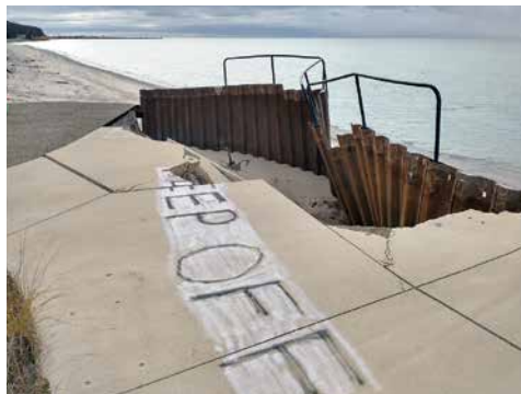
The viewing platform at the Sunset Station in Arcadia was damaged by wave erosion. Photo by S.A. McFerran.
