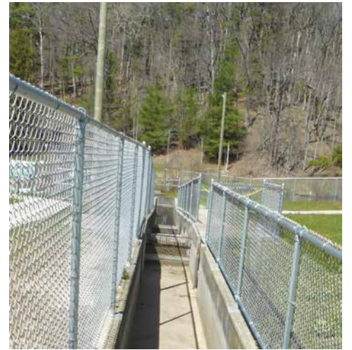
A concrete fish ladder at the Little Manistee River fish weir, next to the dam. During spring and fall salmon runs, the fish ascend the steps to holding ponds where eggs are gathered and fry are raised. Photo by Mark Videan.
