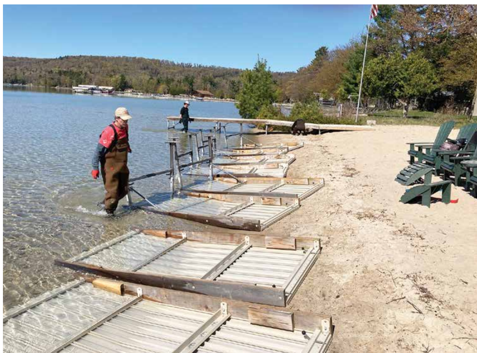
Two members of the Glen Lake Property Management crew lay out dock sections prior to assembly. Photo by Don Sielaff.
