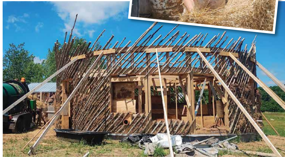
Top: Vonnie Sage is building a light straw-clay house on her Manistee County property. The clay behind her was excavated on site. Above: Vonnie's house takes shape.
