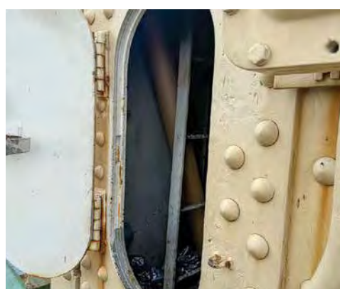
The hatch in the side of the South Tower. Hansen turned his body sideways just to get in.
